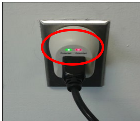
Figure - Picture of Red and Green Lights on the Surge Protector
